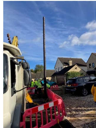
One of the 4 Poles installed by Full Fibre Ltd prior to them halting further work
